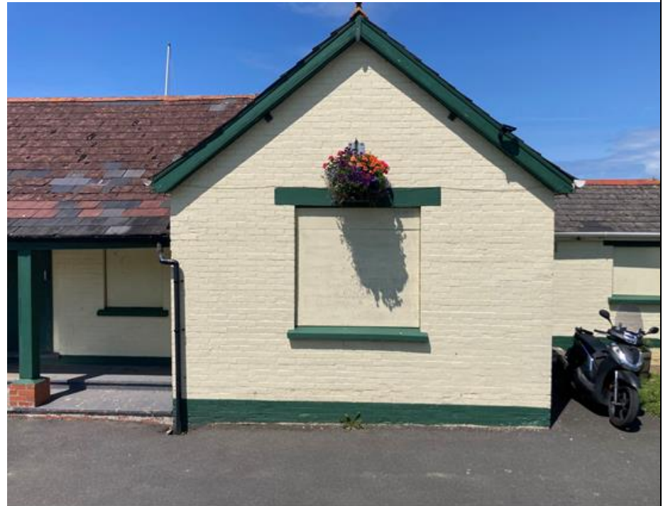
Gable end, right side (Avon Lane end). c1,100mm x 1,100mm either side of window. c1,100mm x 1,100mm within window space.
