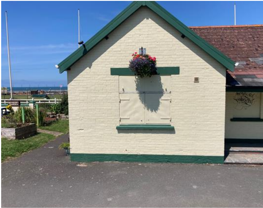
Gable end, left side (Sensory Garden end). c1,100mm x 1,100mm either side of window.
